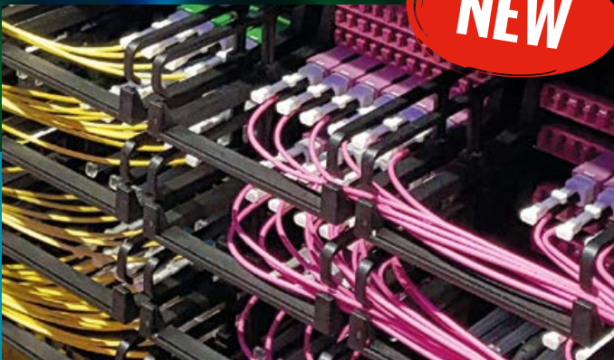
HIGH-DENSITY DATA CENTRE SOLUTION (HD-DCS)
